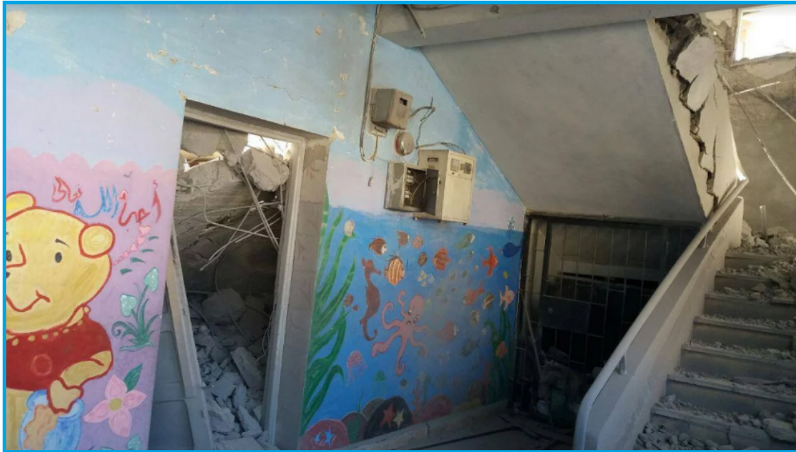
Damages at the Martyr Bashir Abdul Jawad School in the aftermath of an airstrike by Syrian regime forces warplanes in Hamouriya, Damascus suburbs – November 24, 2016
