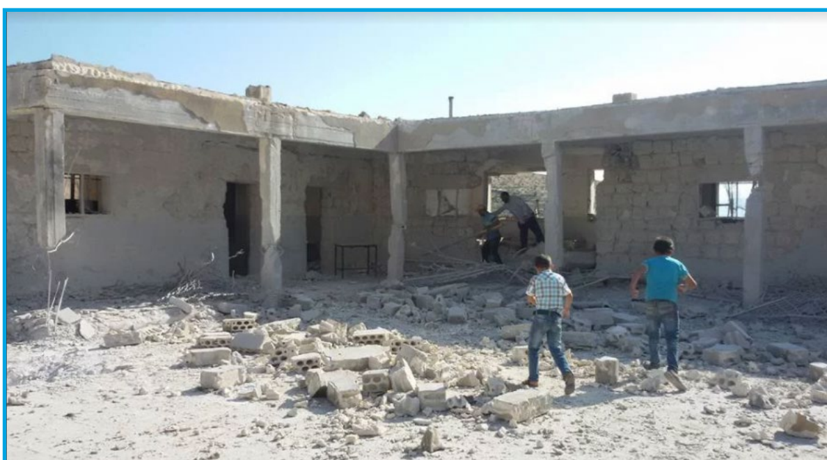
Destruction in the aftermath of a bombing by Syrian regime forces who targeted Ahmad Meghlaj School in Kafr Aweed village, Idlib suburbs – May 31, 2015
